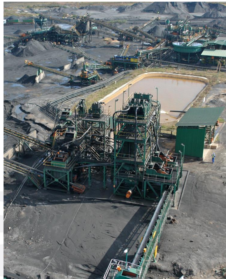
View of Woestalleen wash plant
