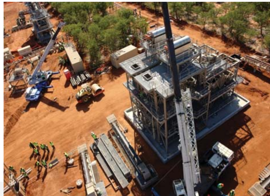
Vele wash plant assembly at site
