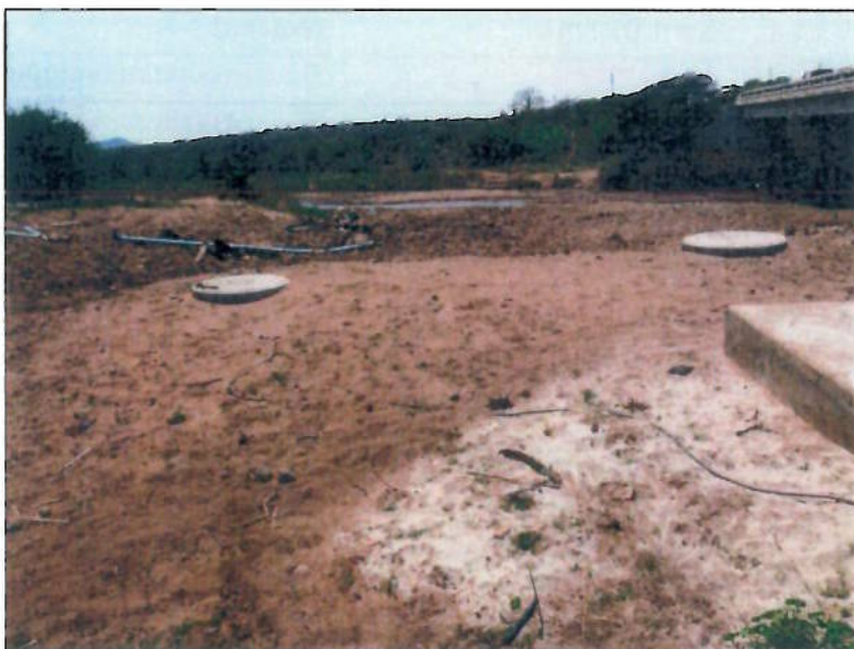
Figure 2 – Damage Alluvial Sand Abstraction System
